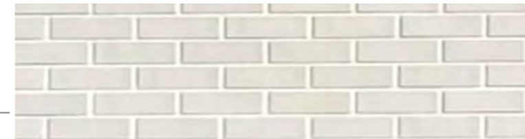
Brick: Platinum White Brick with recessed white Ultra mortar jointing in a stretcher bond.
